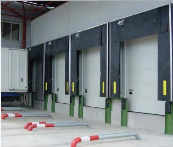
Telesco without hatch in cold-storage facility.
